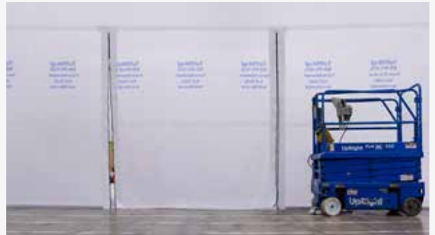
Zipper Doors can be sized large enough for construction vehicles, like scissor lifts.
